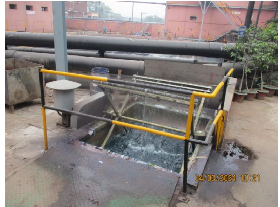
Screening process of ETP.JPG
