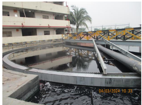
Sedimentation tank of ETP.JPG
