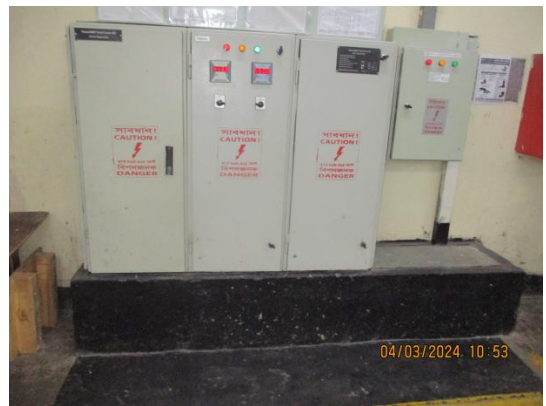
Electric distribution board.JPG
