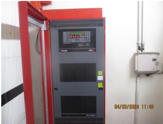
Fire control panel.JPG
