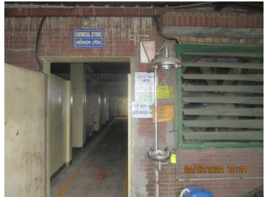
Eye wash station.JPG
