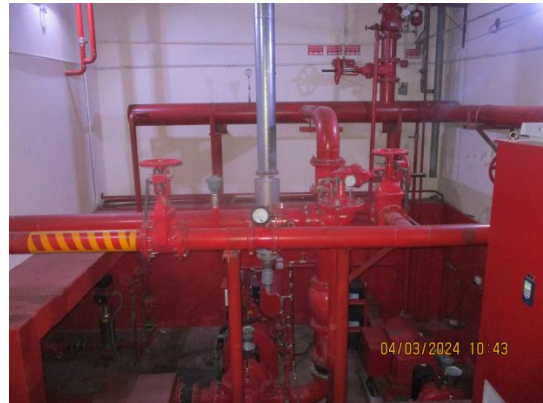
Fire hydrant pump.JPG
