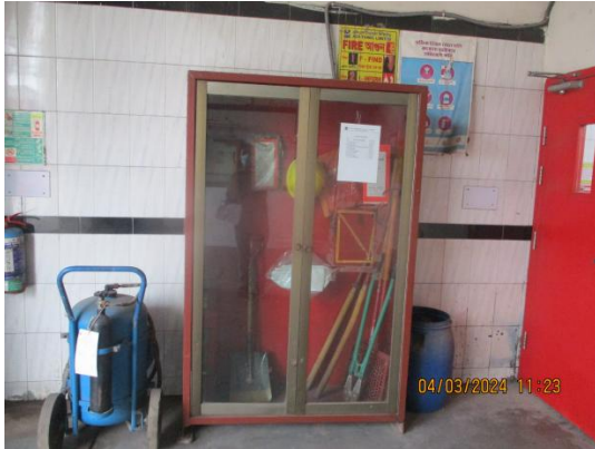
Fire fighting equipment.JPG
