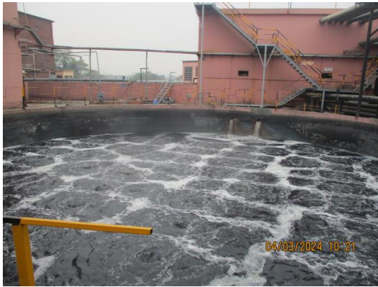
Equalization tank of ETP.JPG
