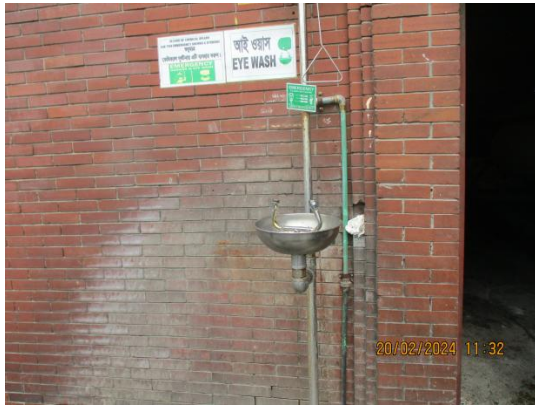
Eye Wash station.JPG
