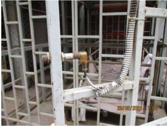
NC Photo-Non-functional interlocks of cargo lift.jpg
