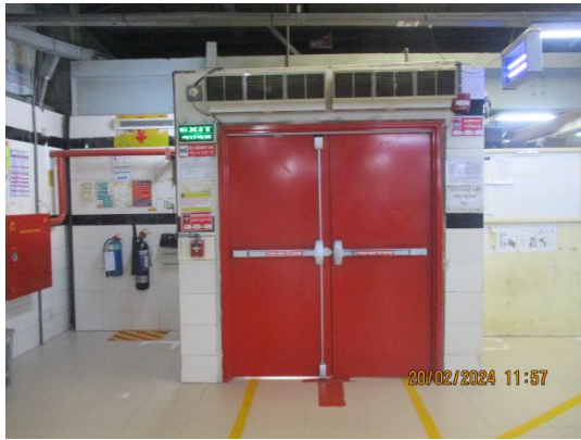
Fire Exit Door.JPG
