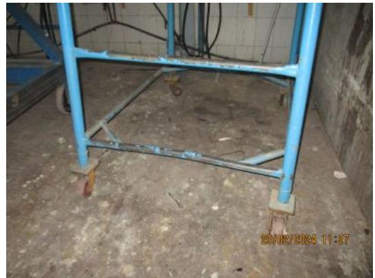
NC Photo-No locking mechanism for platform ladder.jpg
