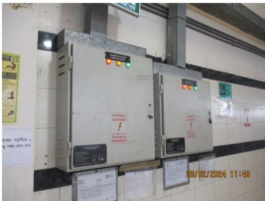
Electric distribution board.JPG
