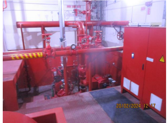
Fire pump room.JPG
