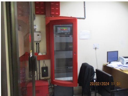
Fire control panel.JPG
